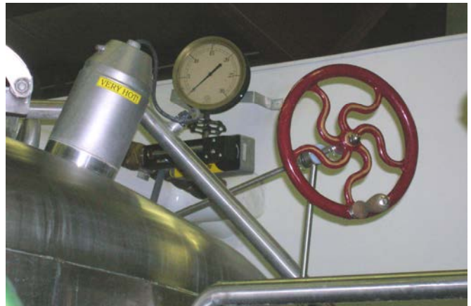
An antique note in a modern facility, this curved spoke wheel opens the steam valve to the brew kettle to control boiling.
