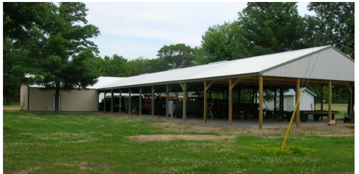
July 5 Sooo, what has changed here? Note the new Ice Cream building tucked in against the picnic shelter. And there is a new 30 ft. extension at the front end of the picnic shelter. Count back 4 posts from the front corner; that is the new addition. A tree was removed to make room.
