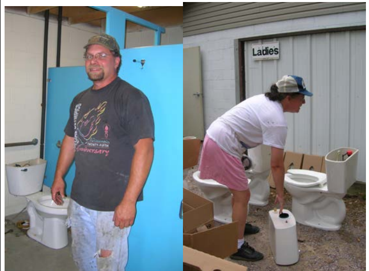
July 5 The grounds were very busy that day. Paul and Heather Kohlwey were hard at work installing new toilets in the restrooms. The new toilets have a 3 inch trap way instead of a 2 inch trap way, so there should not be as many blockages. They are also water saving toilets, and are the high profile type. Easier for the less limber among us...! Thank you to Paul for his expert advice and getting the toilets for us at a reduced price, and thanks to both of them for donating their time. Some new faucets will also be installed, on a trial basis.
