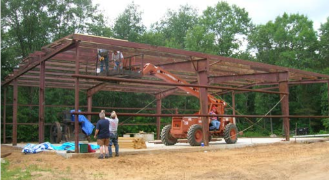
July 5 & July 14 Work on the Fairbanks building is progressing. Workers on the 14 th were Allen Steele, Art Woodward, Pete Holzman and Paul Grotophorst. Jim McGhee contributed feedback before returning to work in the F&J annex.
