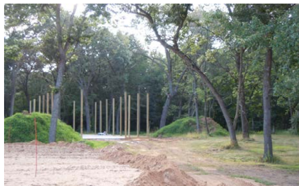
Where is this mysterious place? It looks like the ruins of some ancient mound culture, tucked away in the forest. Oh, wait – it's the Fuller & Johnson Museum Annex construction site last summer.
